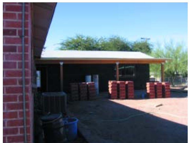
The addition on December 13 was a shell and on January 17 was beginning to look like it belonged to the rest of the house.
